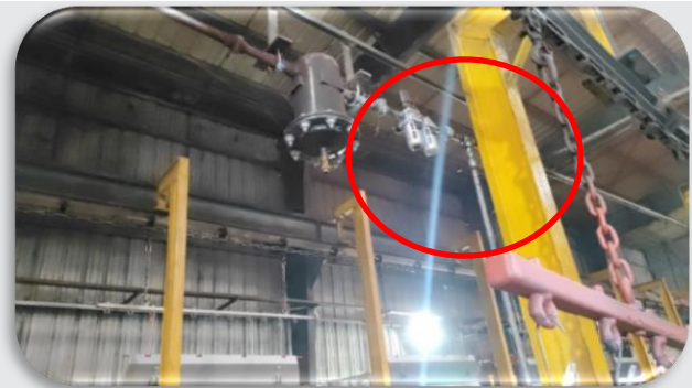
Figure 1: Compressed air leakage point
